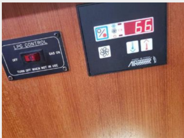
LPG and Air Conditioning Controls
