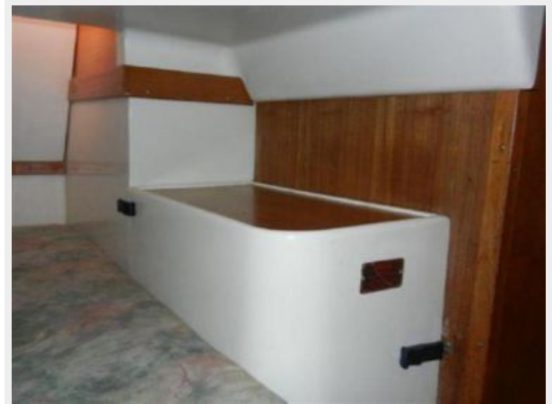
Engine access, aft cabin
