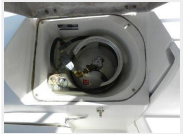
Propane Locker under cockpit seating
