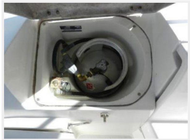
Propane Locker under cockpit seating
