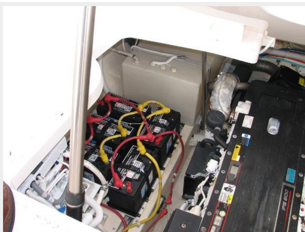
Batteries New in 2015
