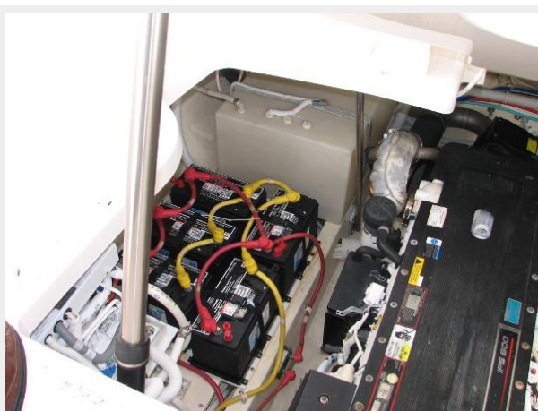
Batteries New in 2015
