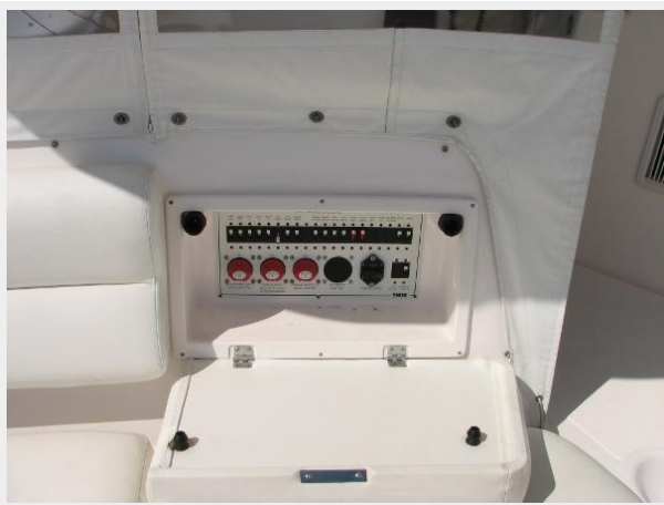
Battery Switches and Circuit Breakers
