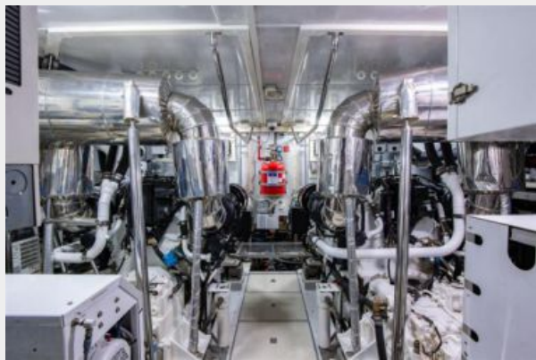
Engine Room Forward
