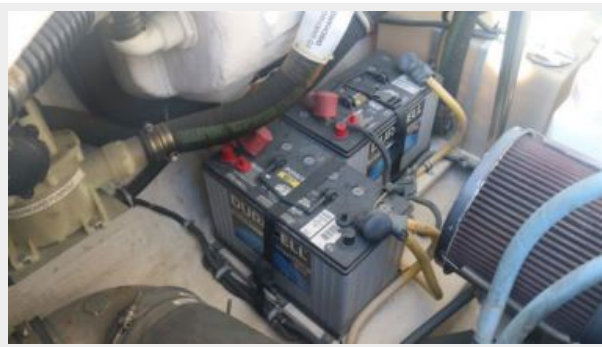
Port AGM Battery Bank
