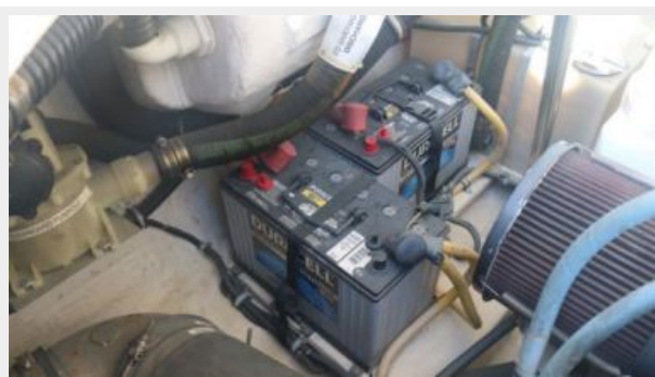
Port AGM Battery Bank
