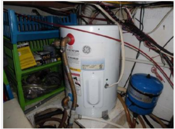
GE Water Heater
