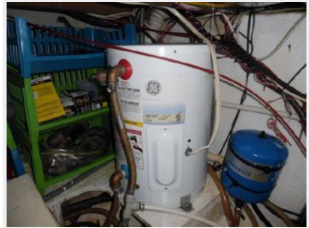
GE Water Heater
