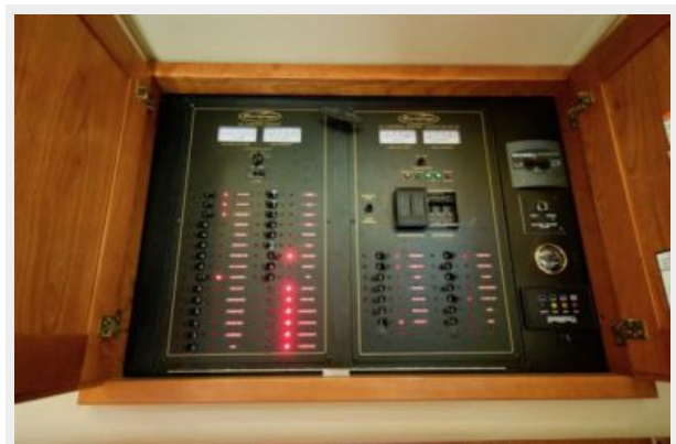
Main Distribution Panel
