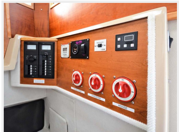
Electrical Panel and Controls
