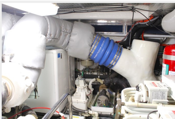
Engine Room Starboard 2
