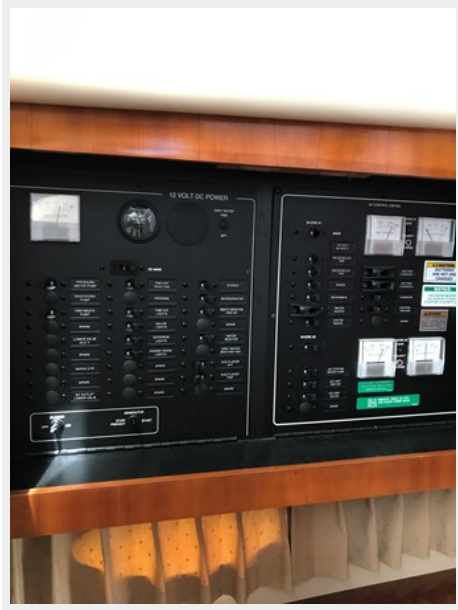
360 Carver SS - Distribution Panel
