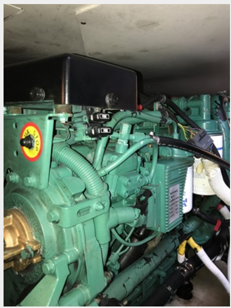
360 Carver SS - Engine Room
