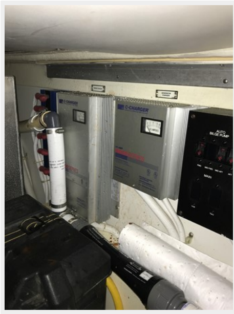
360 Carver SS - Engine Room Battery Chargers
