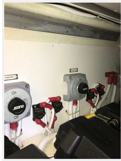
360 Carver SS - Engine Room Battery Switches
