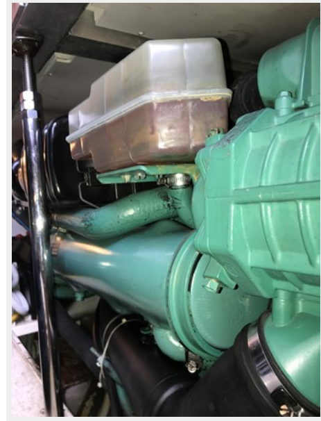
360 Carver SS - Engine Room
