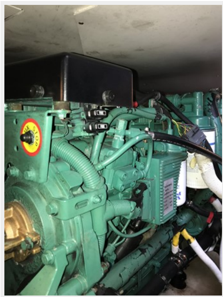
360 Carver SS - Engine Room
