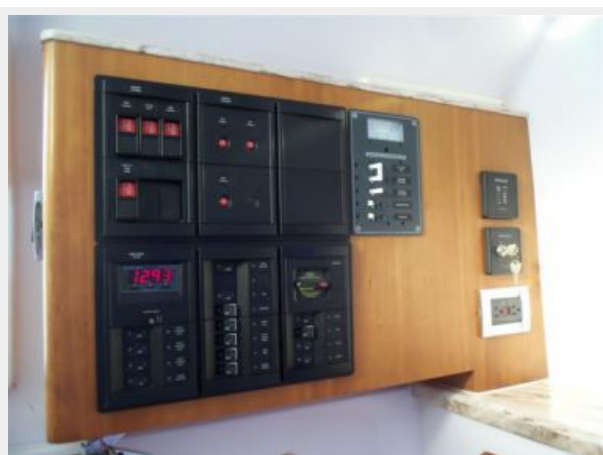
Console Electrical Panel
