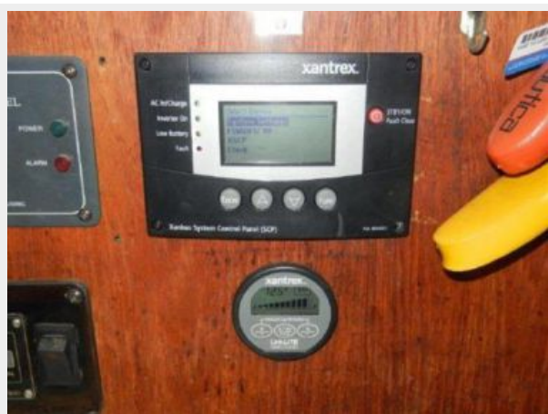
Xantrex panel for inverter and battery monitor
