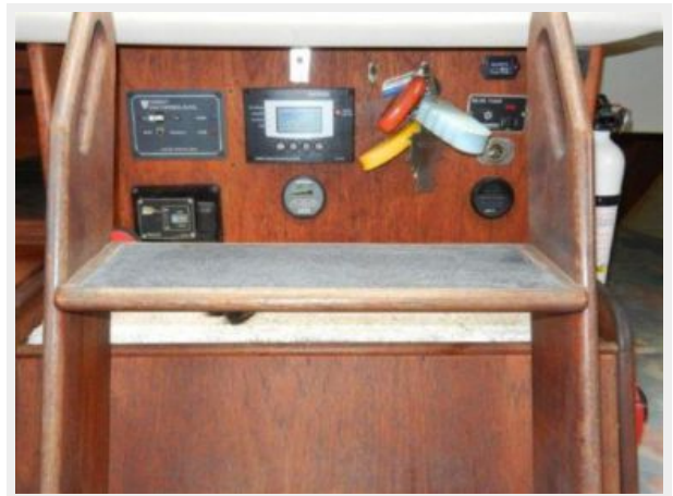
Instruments behind companionway ladder
