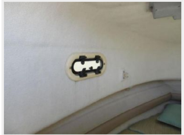
Interior Port - No Leaks
