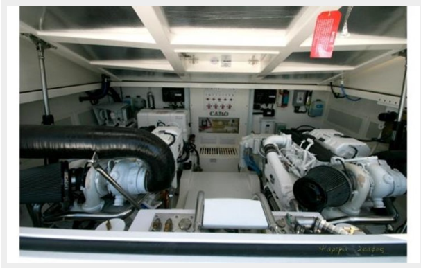
Engine Room Looking Forward
