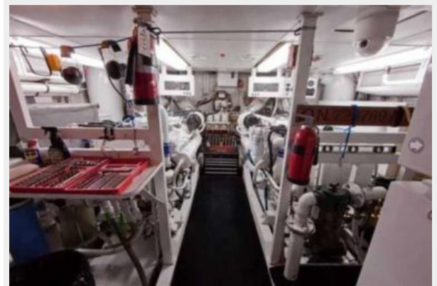
Engine Room Looking Aft
