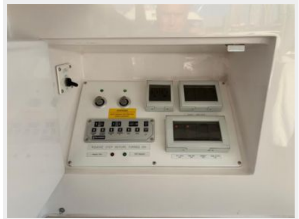
Aft Deck Lighting / Passerelle Cabinet
