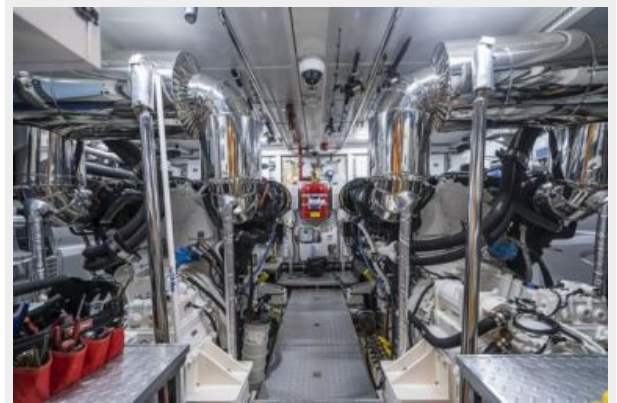
Engine Room Forward
