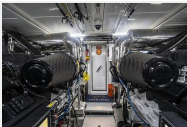
Engine Room Aft
