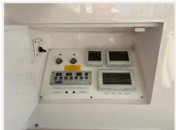
Aft Deck Lighting / Passerelle Cabinet
