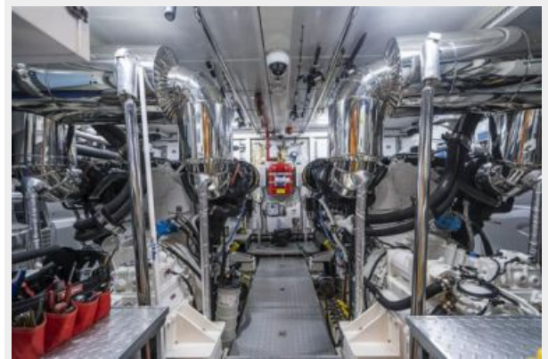
Engine Room Forward
