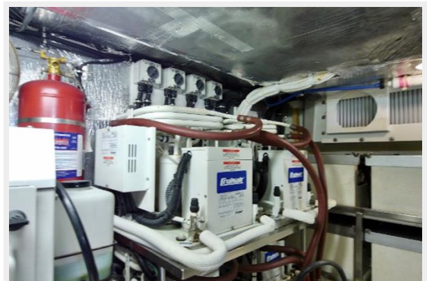
Air Conditioning Compressors
