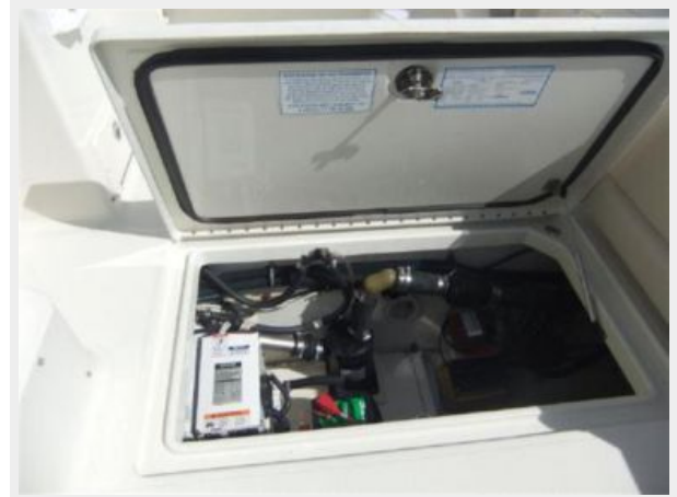
Cockpit generator compartment
