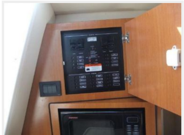
Breaker panel in cabin
