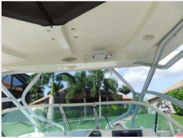
Over heat electronics box
