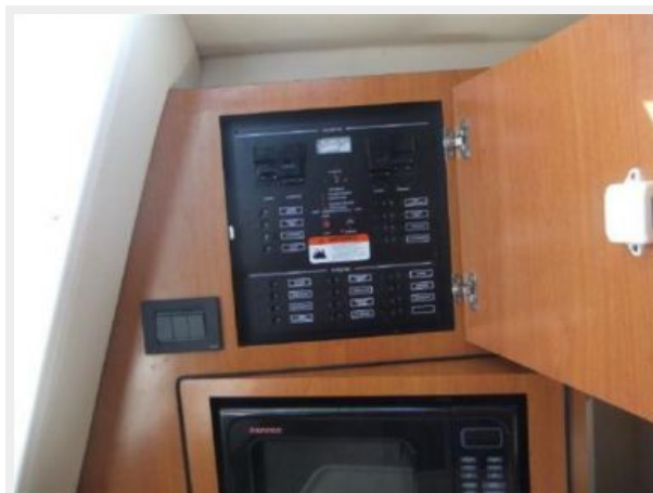
Breaker panel in cabin
