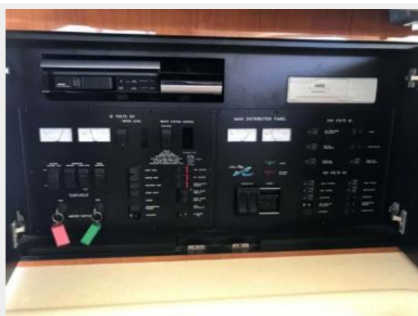
Main Distribution Panel
