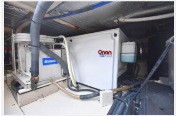
2004 Sea Ray 48 Sedan Bridge - Engine Room
