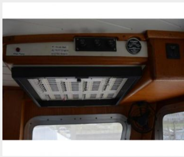
Overhead AC DC Panels
