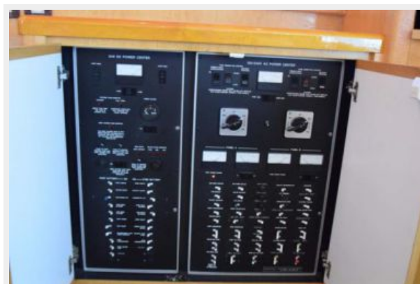
AC and DC Panel Detail
