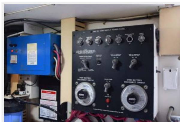
DC Power Panel
