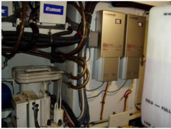
Forward Starboard Engine Room
