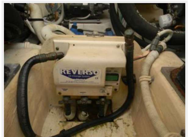
Oil Exchanger System
