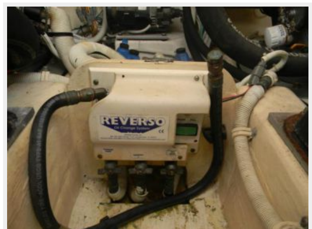
Oil Exchanger System
