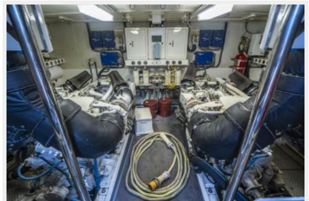
Rear Full Beam Engine Room
