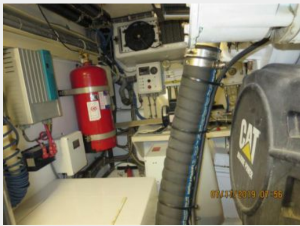
2002 60' Hatteras Convertible Engine Room
