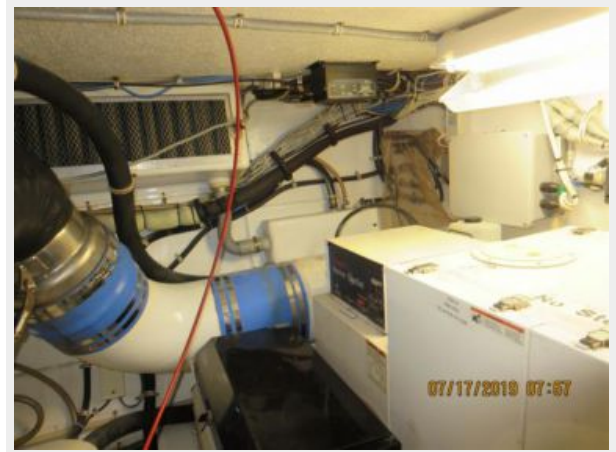
2002 60' Hatteras Convertible Engine Room
