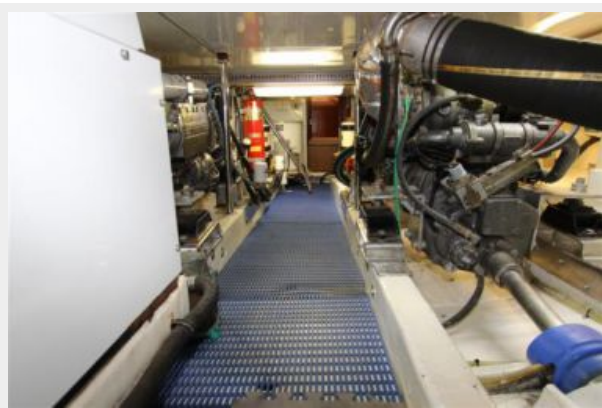
Engine Room Looking Forward
