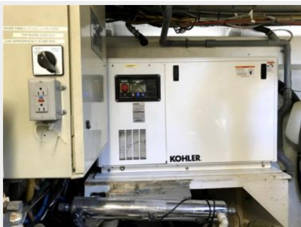
NEW generators - & 500 hrs
