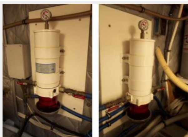
Port and Starboard Racor Filters With Vacuum Gauges
