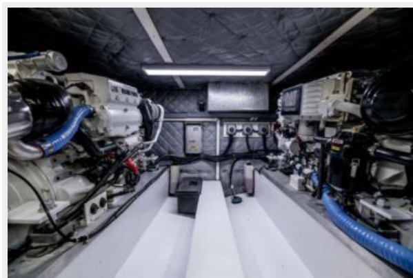
Engine Room forward
