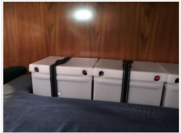
solar battery bank
