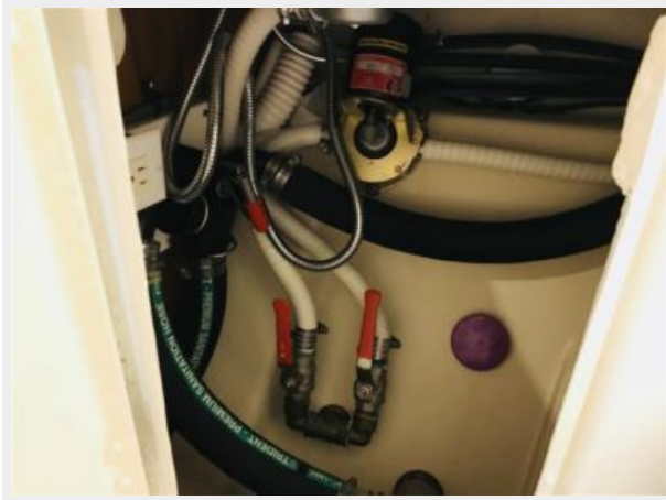
ensuite plumbing access
