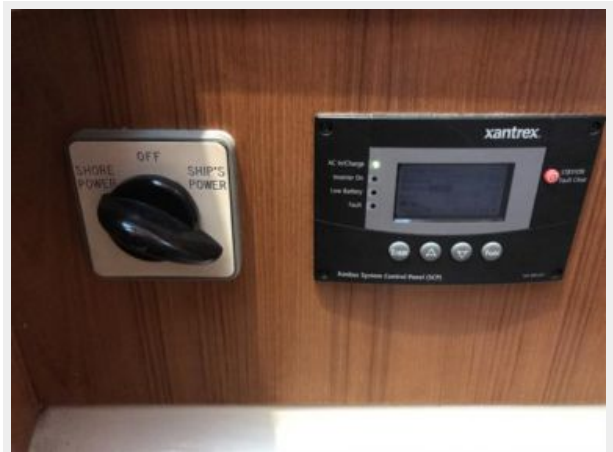
battery charger controls
