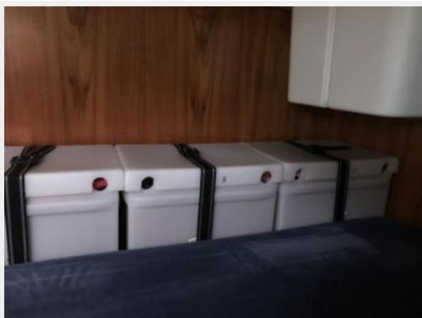
solar battery bank
