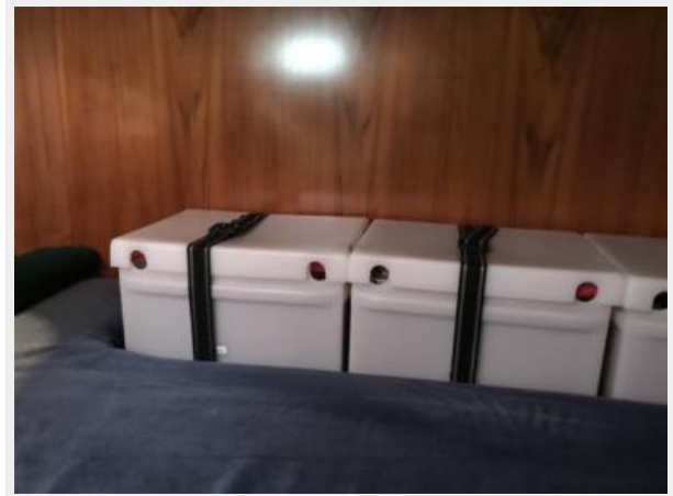
solar battery bank
