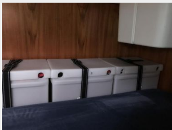
solar battery bank
