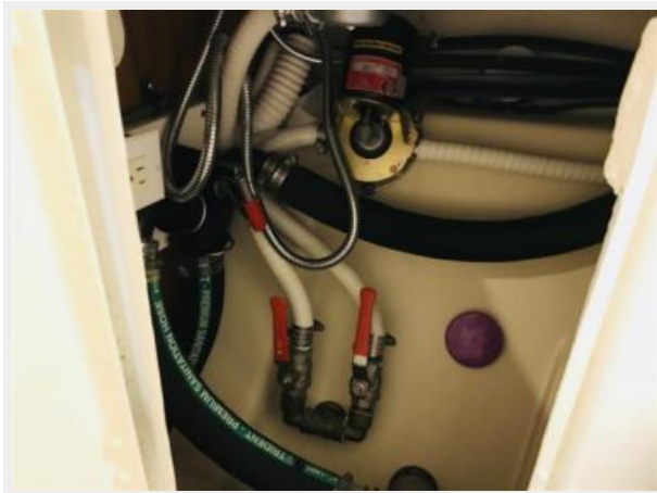
ensuite plumbing access
