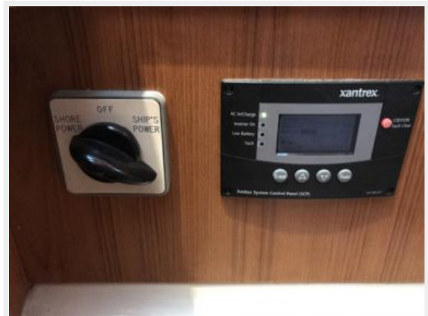
battery charger controls
