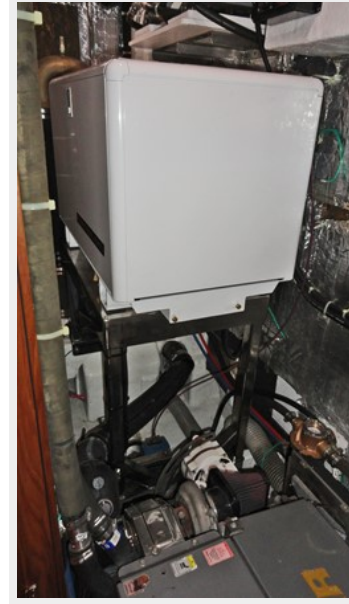
Engine Room, Aft
