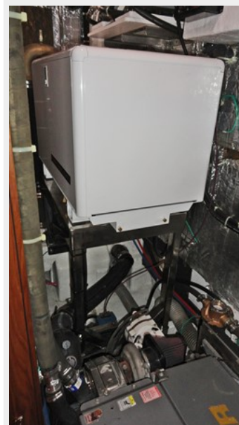
Engine Room, Aft
