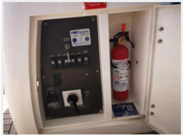
Aft Deck Battery Switch and Fire Extinguisher
