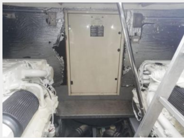
Engine Room Crew Access
