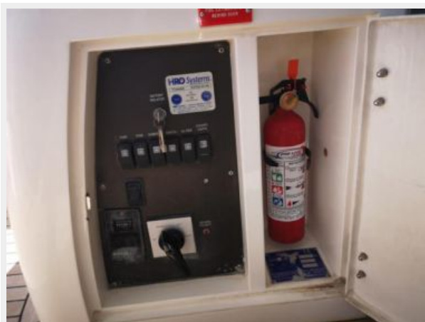
Aft Deck Battery Switch and Fire Extinguisher
