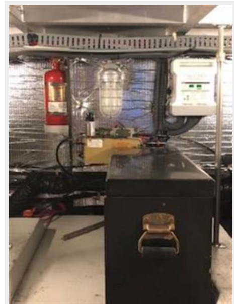
#35 Battery Charger & Fire Suppression
