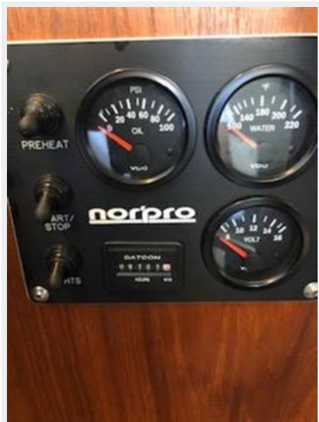
#38 Generator Instrument Cluster
