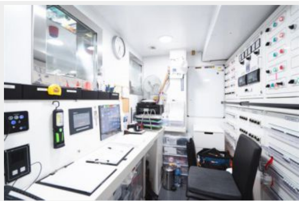
Engine Control Room
