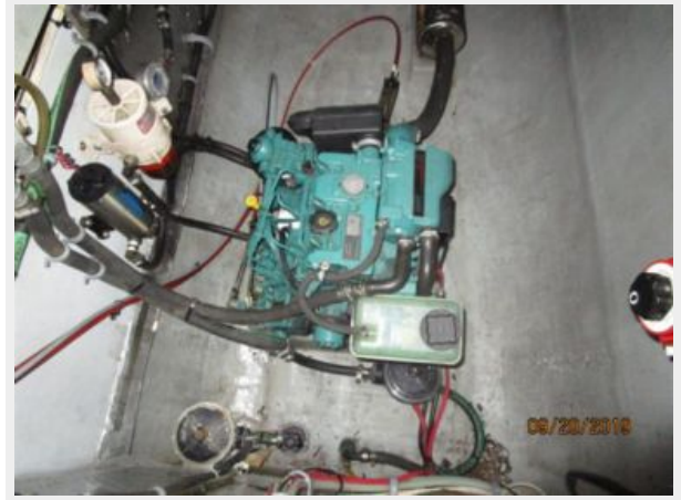
52 Zep Tepi port engine room1 9-20-19
