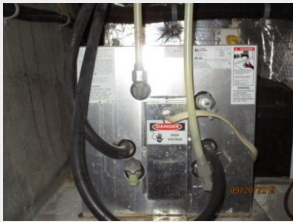
56 Zep Tepi water heater 9-20-19(1)
