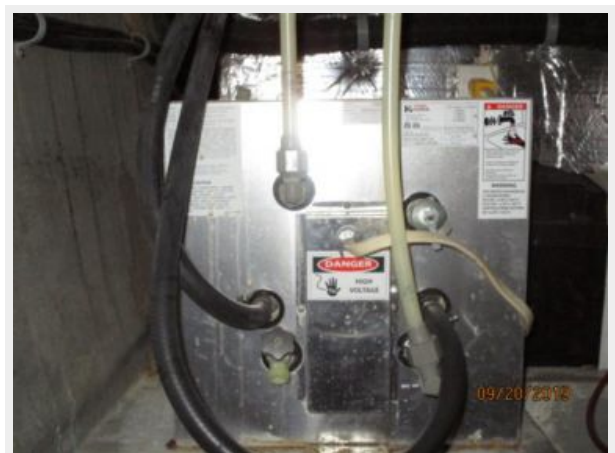
56 Zep Tepi water heater 9-20-19
