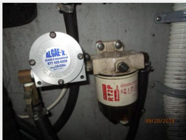
55 Zep Tepi generator fuel filter 9-20-19
