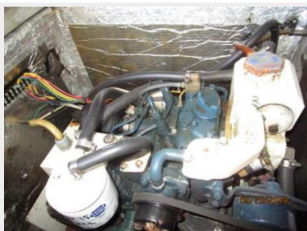
57 Zep Tepi generator 9-20-19
