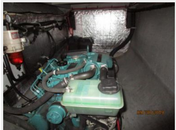
53 Zep Tepi port engine room2 9-20-19
