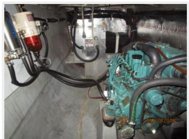
52 Zep Tepi stbd engine room2 9-20-19
