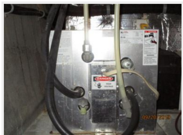
56 Zep Tepi water heater 9-20-19
