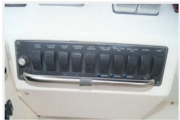
303 Bridge 12v Panel
