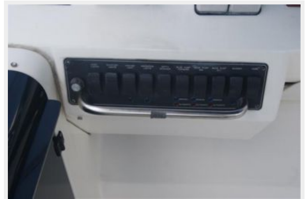
121 Bridge 12v Panel
