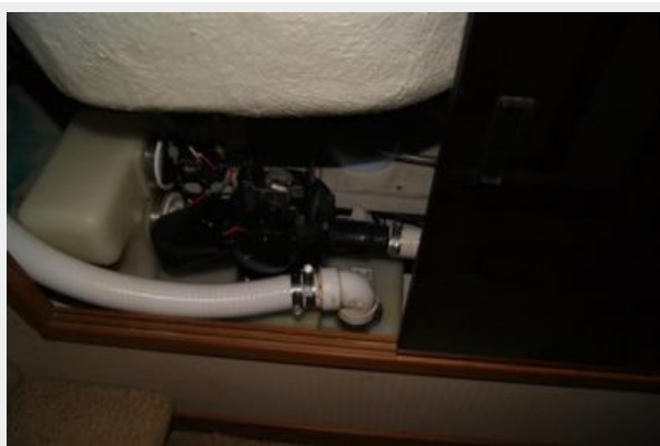
326 Holding Tank Vacuum Generator
