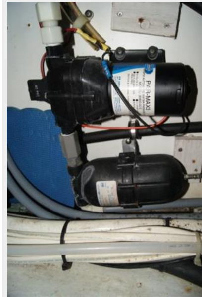
336 FW Pump & Accumulator
