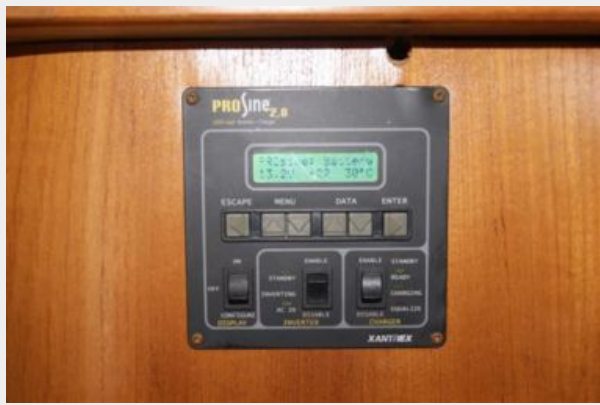
320 PH Battery Monitor
