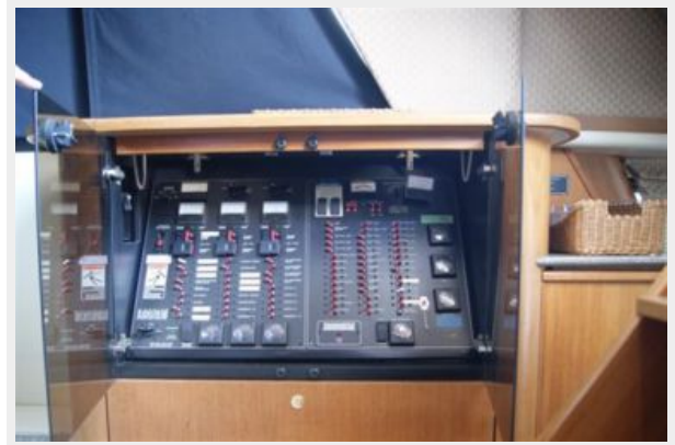
220 Electrical Distribution Panel
