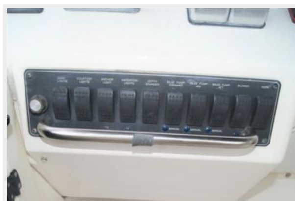
303 Bridge 12v Panel
