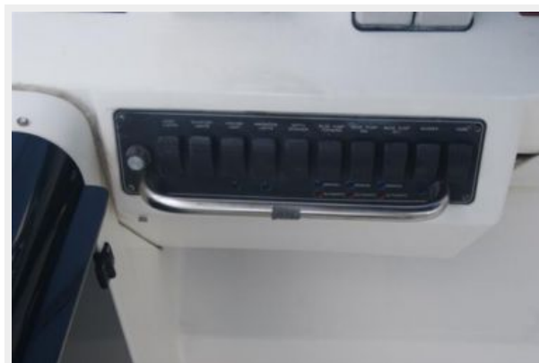
121 Bridge 12v Panel
