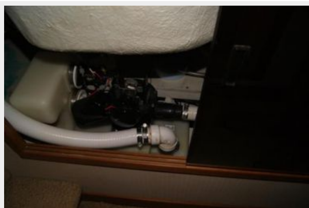
326 Holding Tank Vacuum Generator
