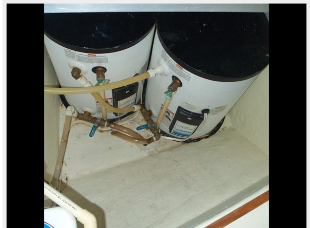
Water Heaters Below VIP
